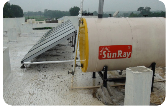
Solar Water Heating System
