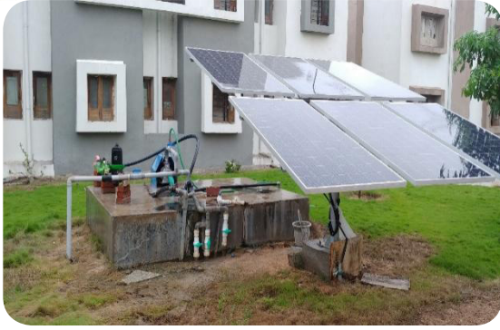
Solar Water Pumping System
