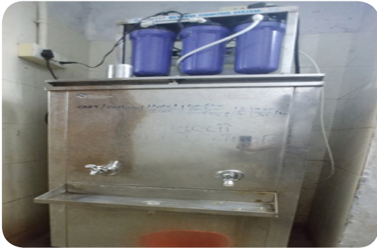
Drinking water with RO facility
