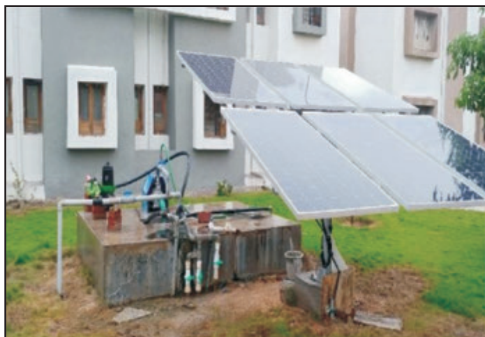
Solar Water Pumping System
