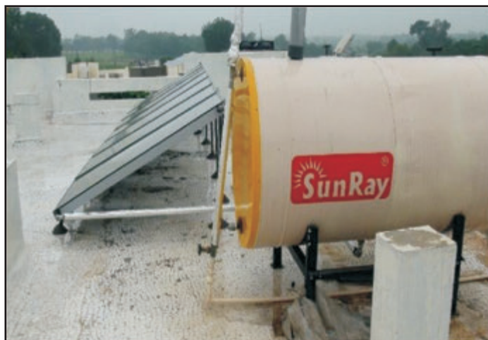
Solar Water Heating System
