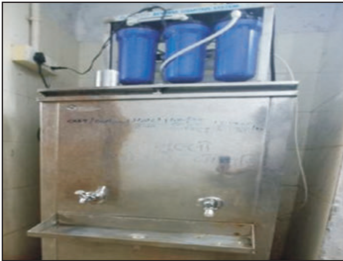
Drinking water with RO facility
