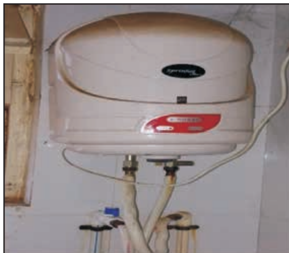
Electric Geyser for water heating
