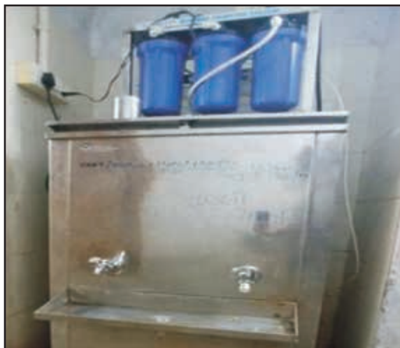
Drinking water with RO facility
