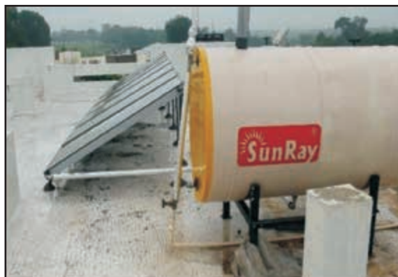
Solar Water Heating System
