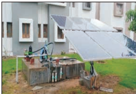
Solar Water Pumping System
